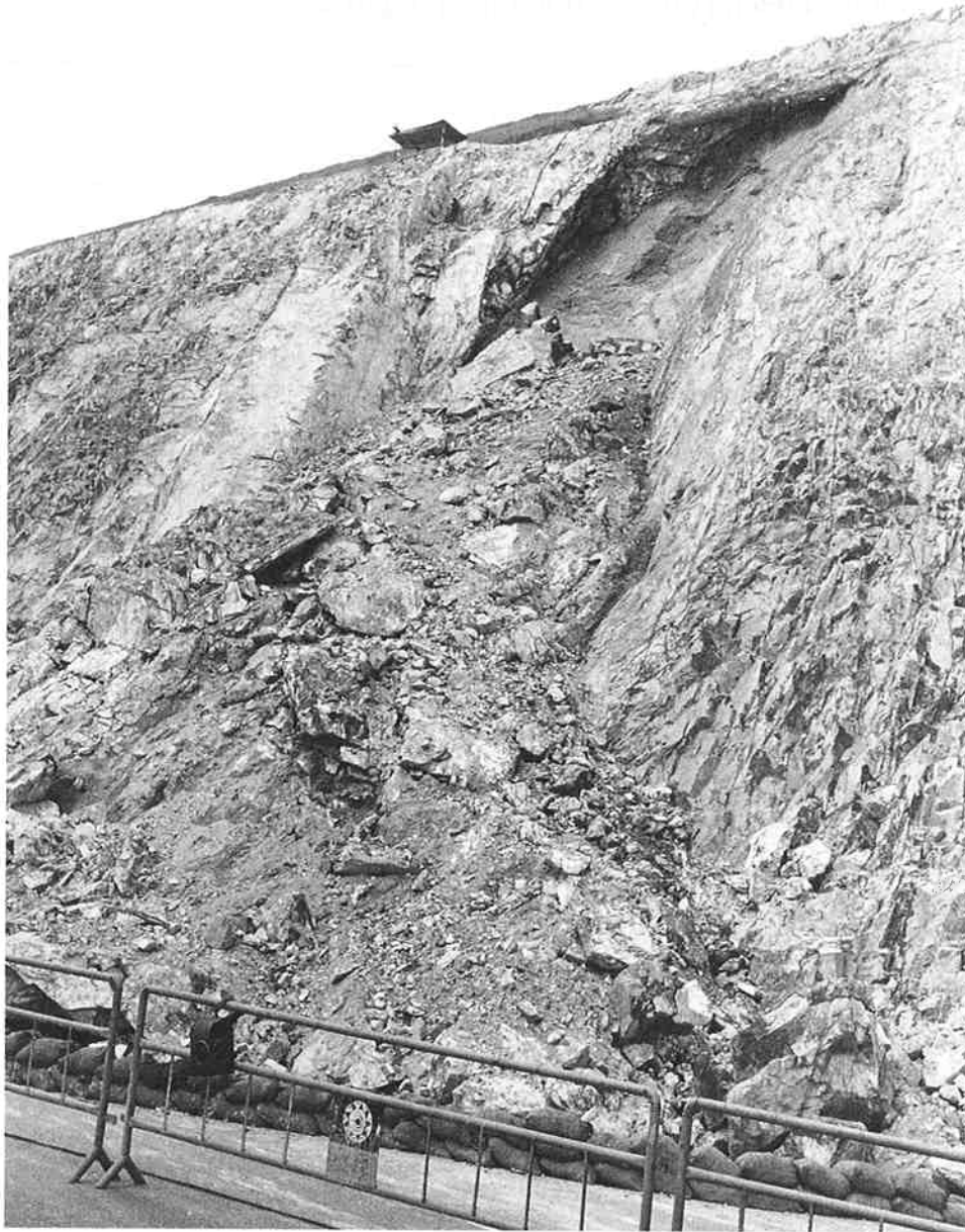
Fig. 1 Complex slope failure in weak rock mass, Tsing Yi Island, Hong Kong
